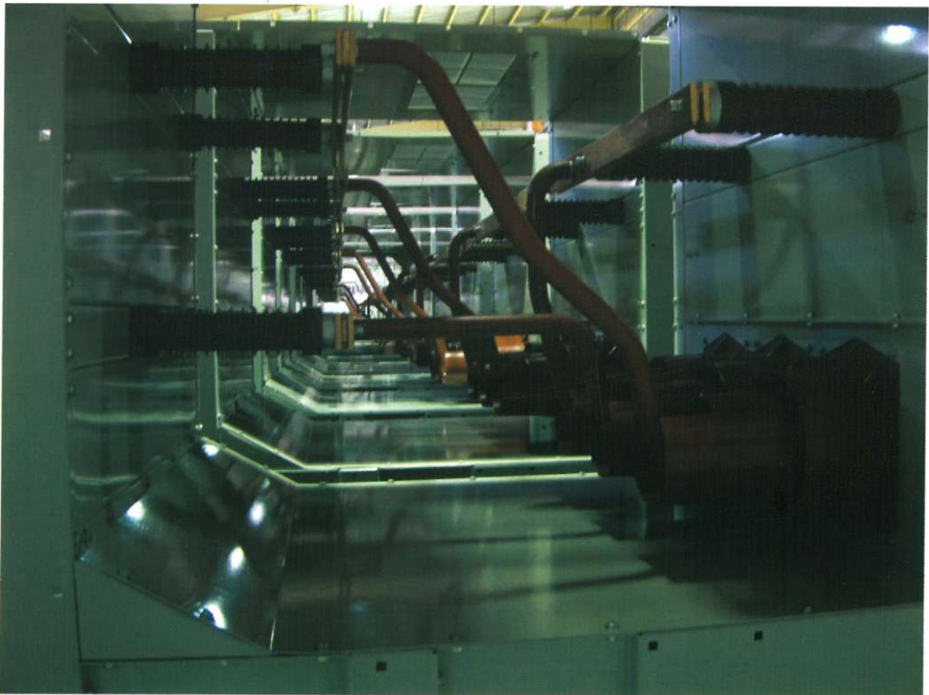
View from Busbar Compartment
