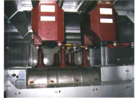
Bus-Bar Compartment with PT
